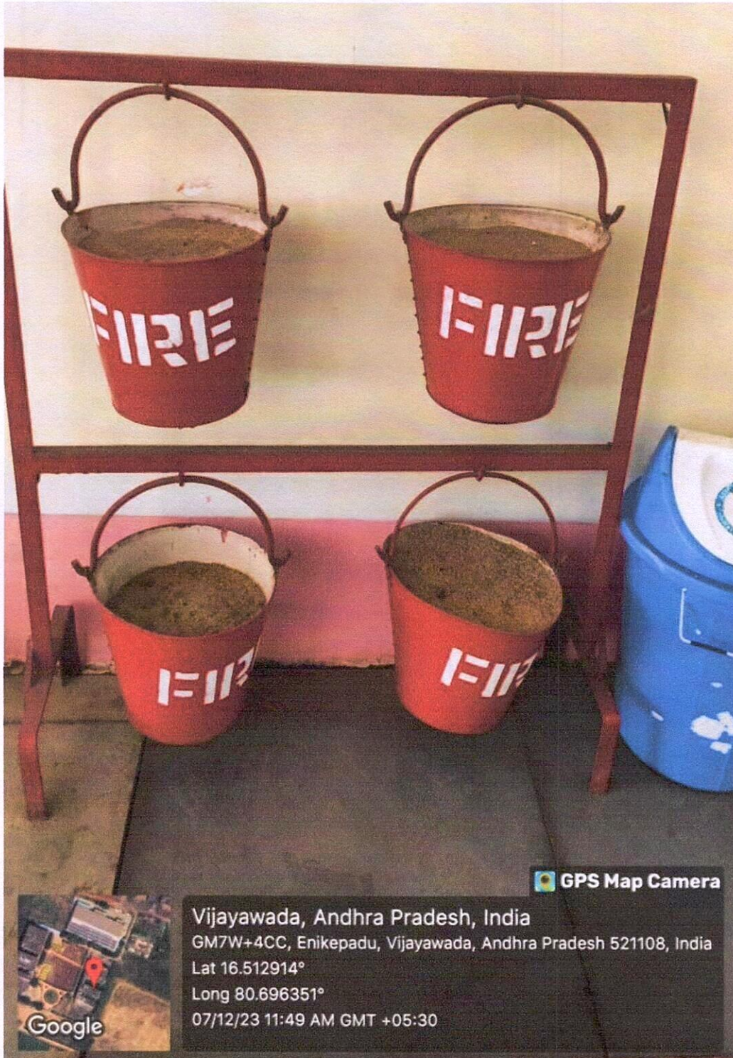
FIRE SAFETY SAND BUCKET
